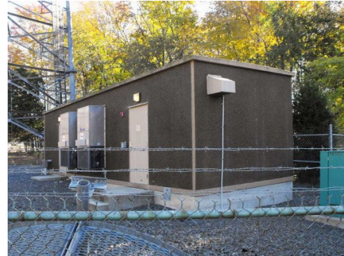
Figure 8: Example precast communications shelter
